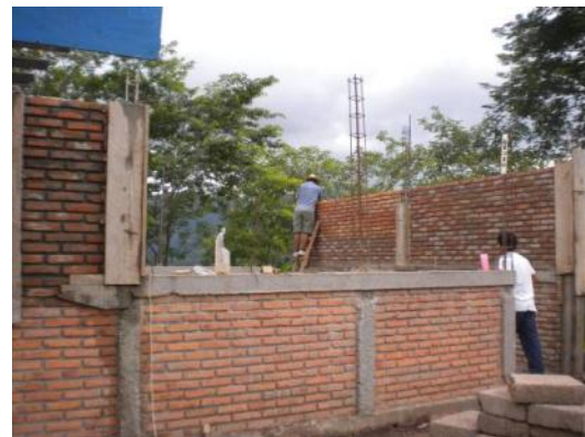
Laguna Seca Preschool walls go up, adjacent to the community's elementary school.
